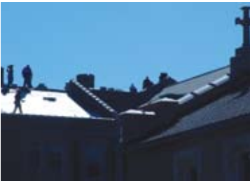
Construction workers complete roof repairs to the Ursuline Academy of New Orleans.
